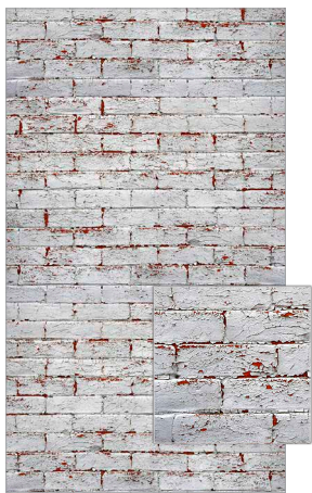
Brick Wall, Peeling Paint
